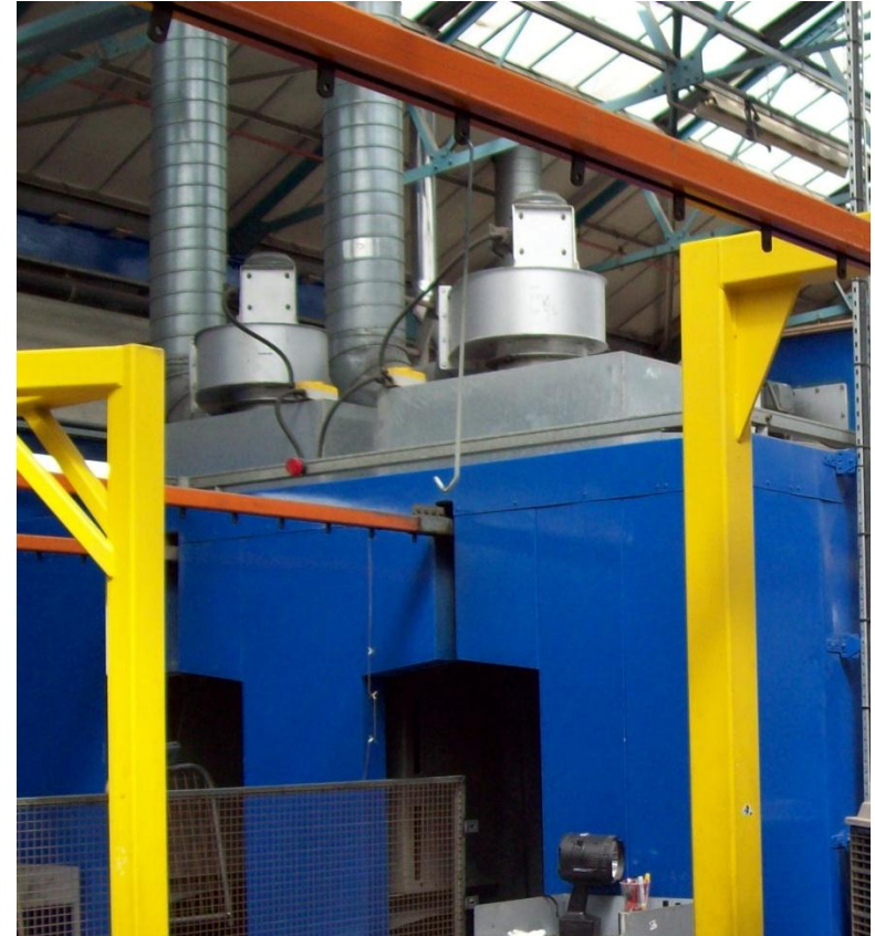
TOTAL LOSS VESTIBULE EXTRACTION SYSTEM
